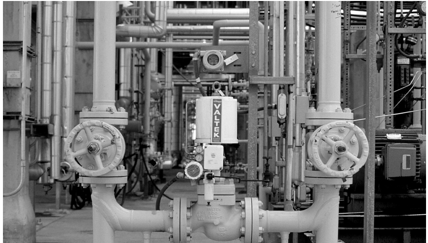
This 8-inch back-pressure control valve operates in a liquid hydrocarbon plant with a 580 psi/40 bar upstream pressure
