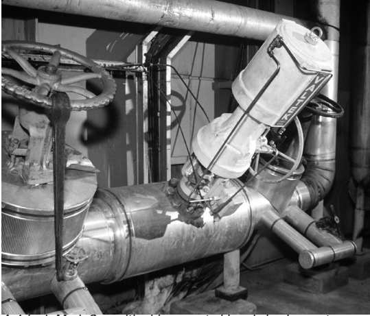
A 4-inch Mark One with side-mounted handwheel operates a boiler feedwater system at a pulp plant.
