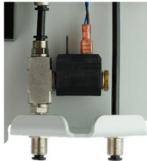
Figure: View of the solenoid valve (no indicator bottle installed)
